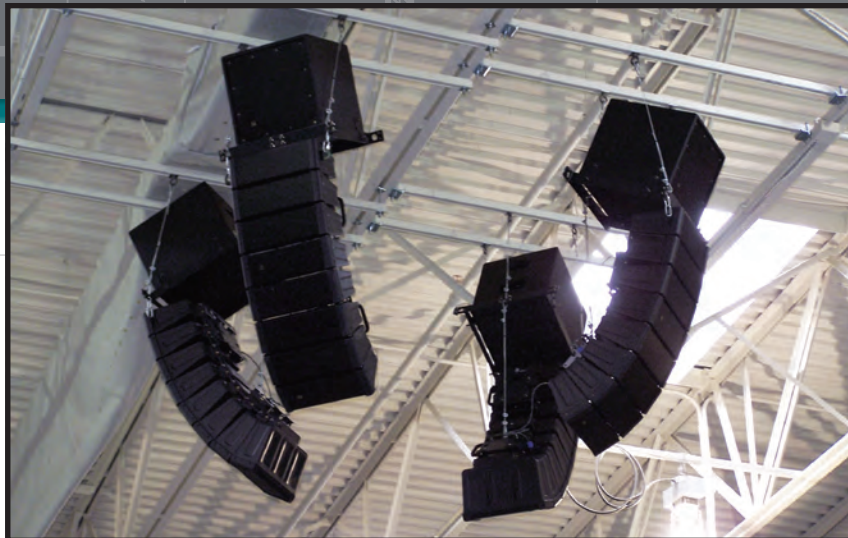
Kamiak High School, Gymnasium Sound System
