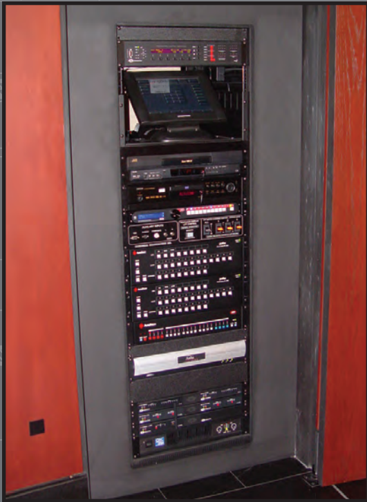
Integrated Equipment Rack
