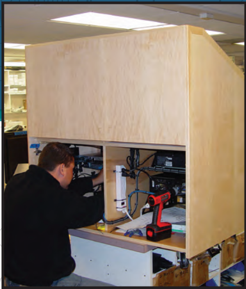
All head-end electronics are installed into their cabinets or equipment racks before leaving DCI.
